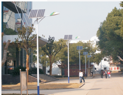
Solar Street Light (Park)
